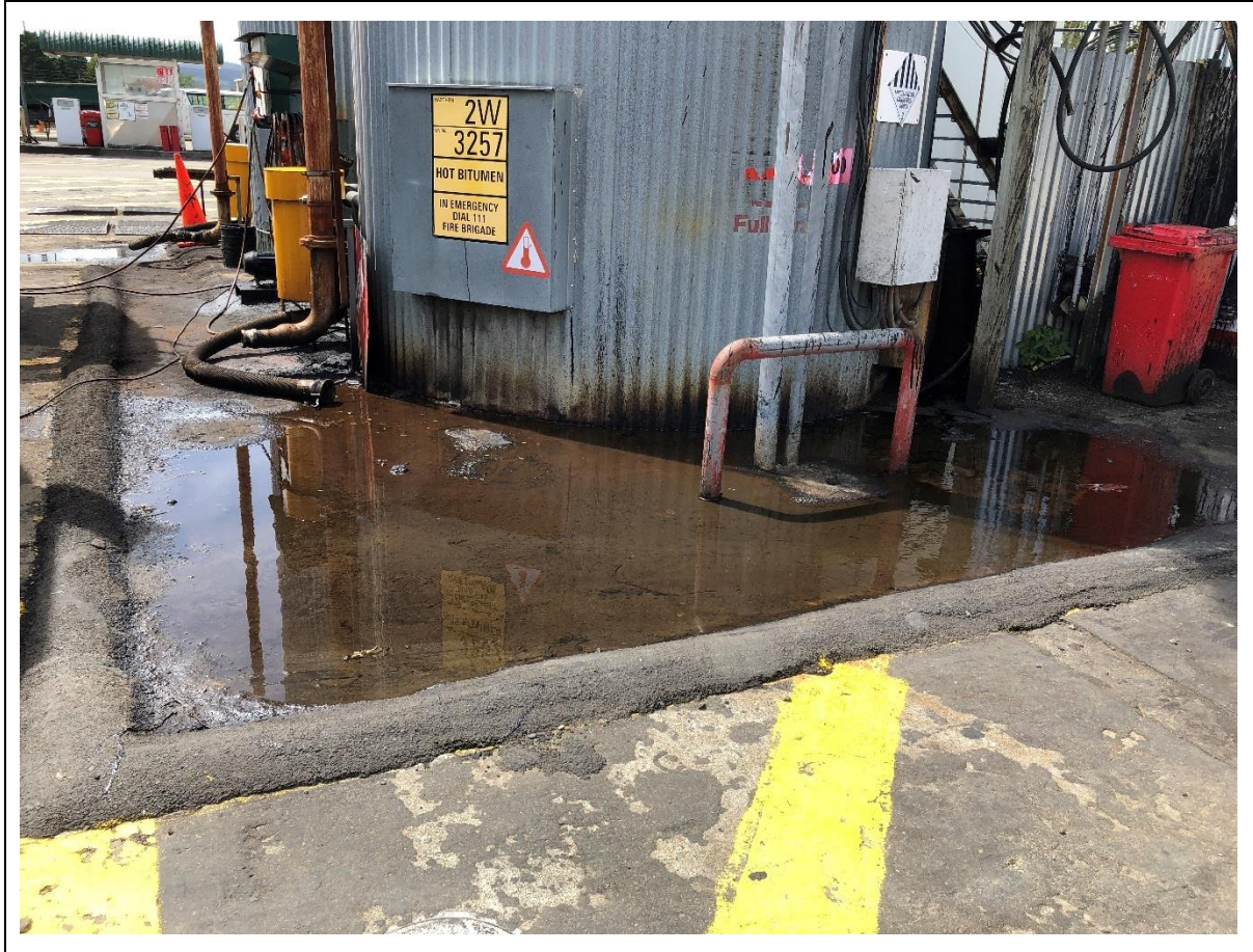
Photograph 9: Bunding surrounding bitumen storage tanks
