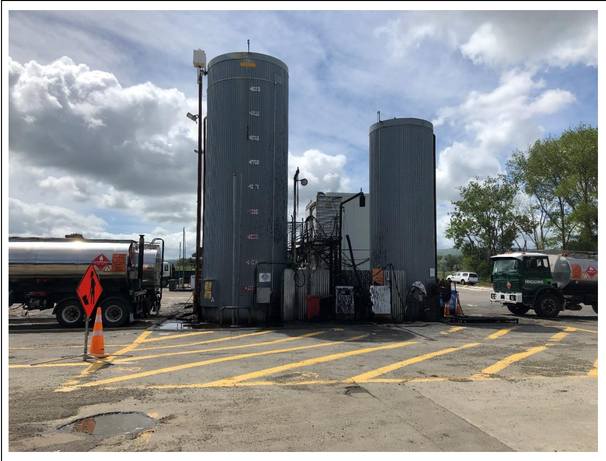
Photograph 8: Large bitumen storage tanks on Higgins site (third tank not visible, behind tank to left of image)
