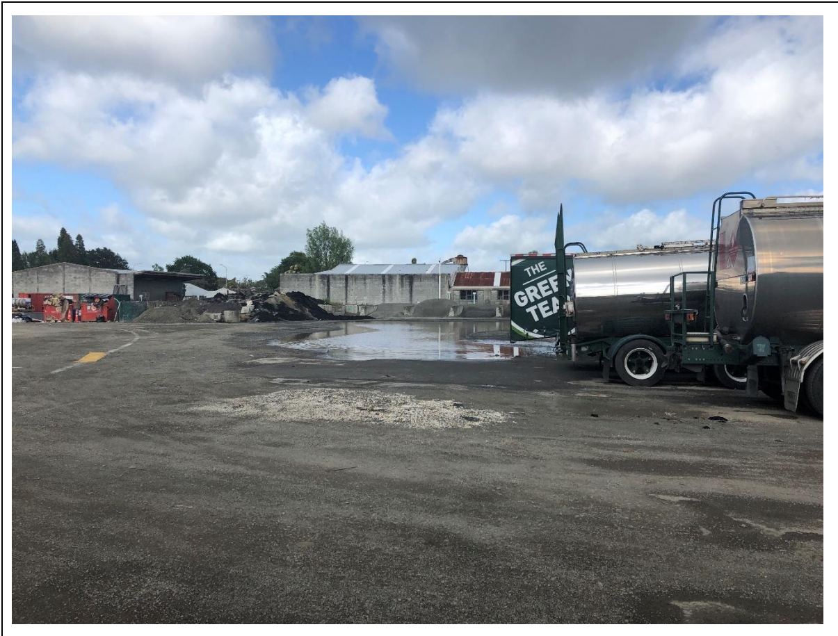
Photograph 12: Ponding of water observed in the middle of the Higgins site
