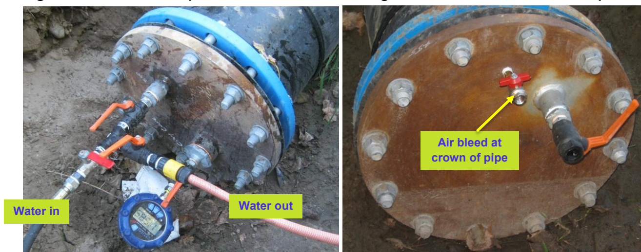
Figure D1: View of end plate and connections. Figure D2: View of the other end plate.
