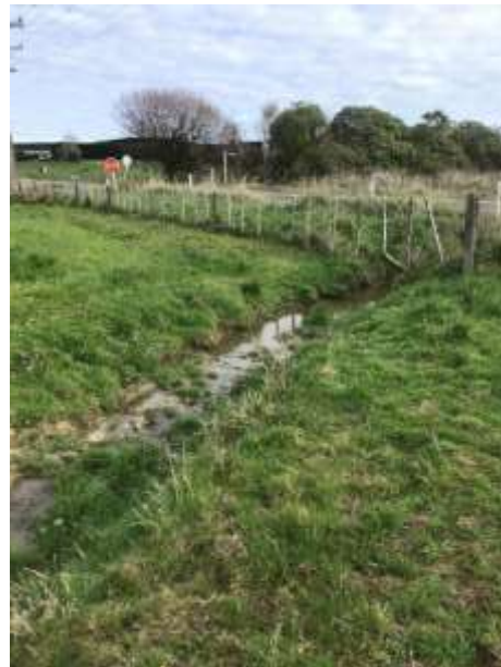
Image 2: Ephemeral flow path immediately upstream of Clevely Line. Note the ponding upstream of the small culvert.
